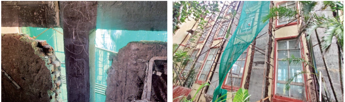
Before applying micro concrete, corroded materials and steel bars should be cleaned and coated.
